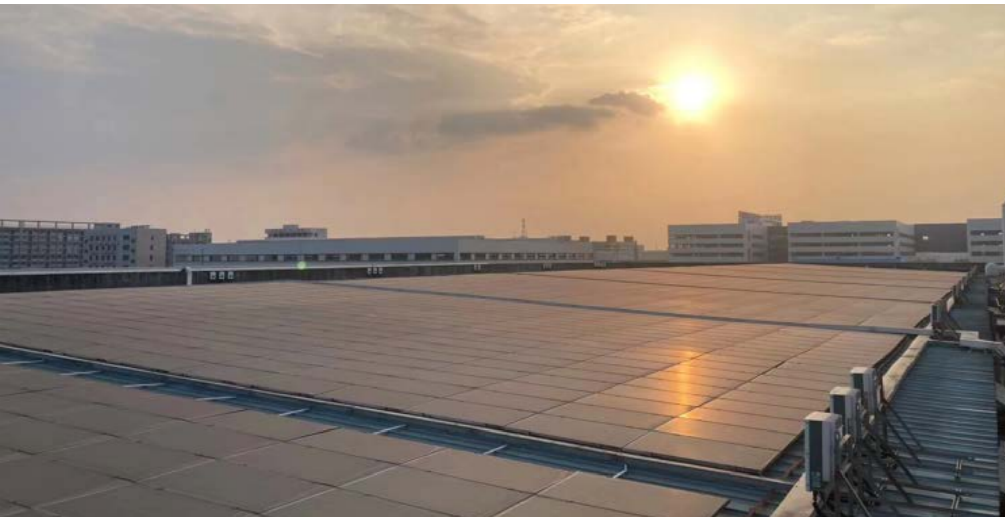
Foshan Base PV Generation Project on Rooftops
