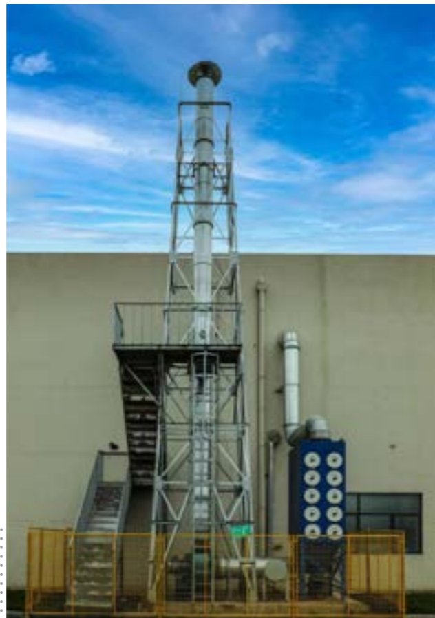
Waste Gas Treatment Facilities
