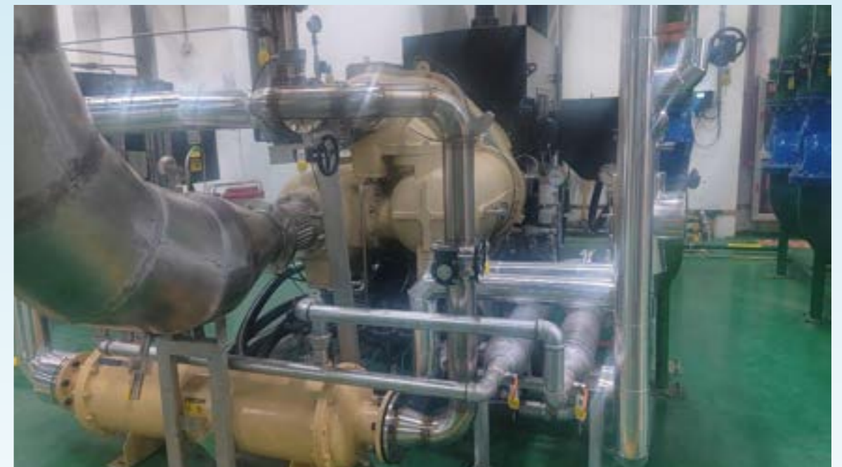
Heat Transport Pipelines
