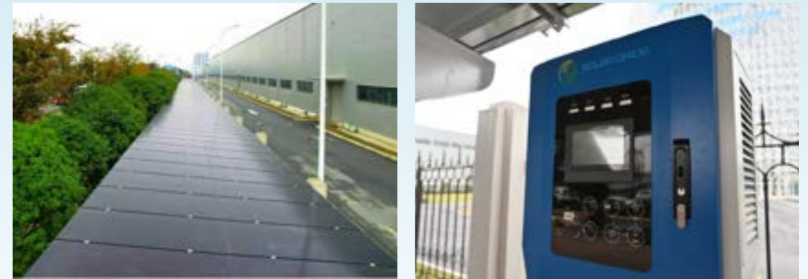
PV Car Parking Shed
